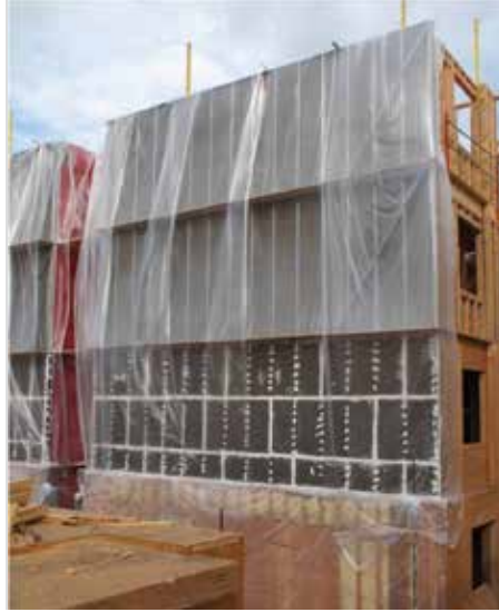
This photo shows how a multi-story wood building can be protected from the elements.
