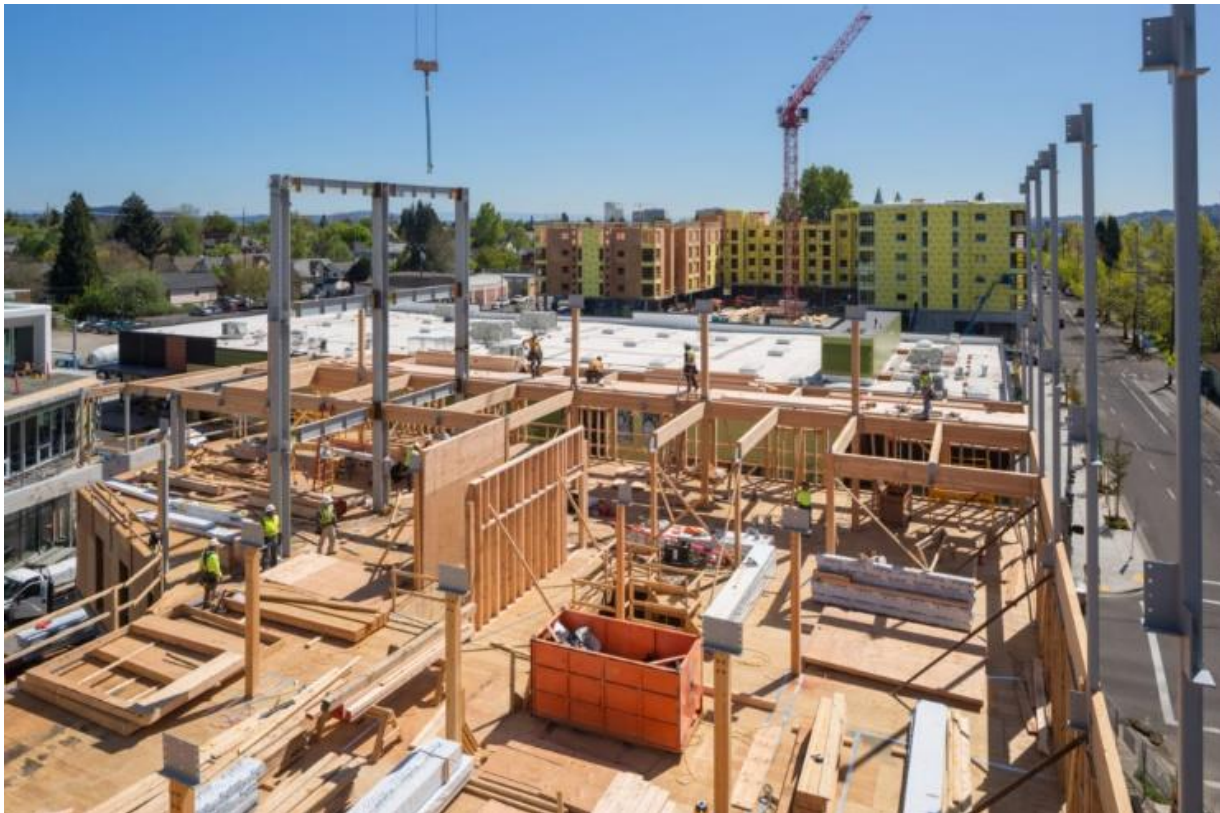
One North's West Building, which was completed last year, pushes the expectations of commercial construction through use of wood.
