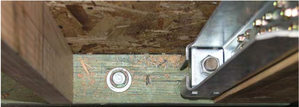
Figure 16. Splitting of bottom plate (Wall H1)
