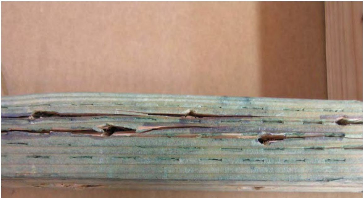
Figure 17. Splitting on narrow face of bottom plate (Wall H1)
