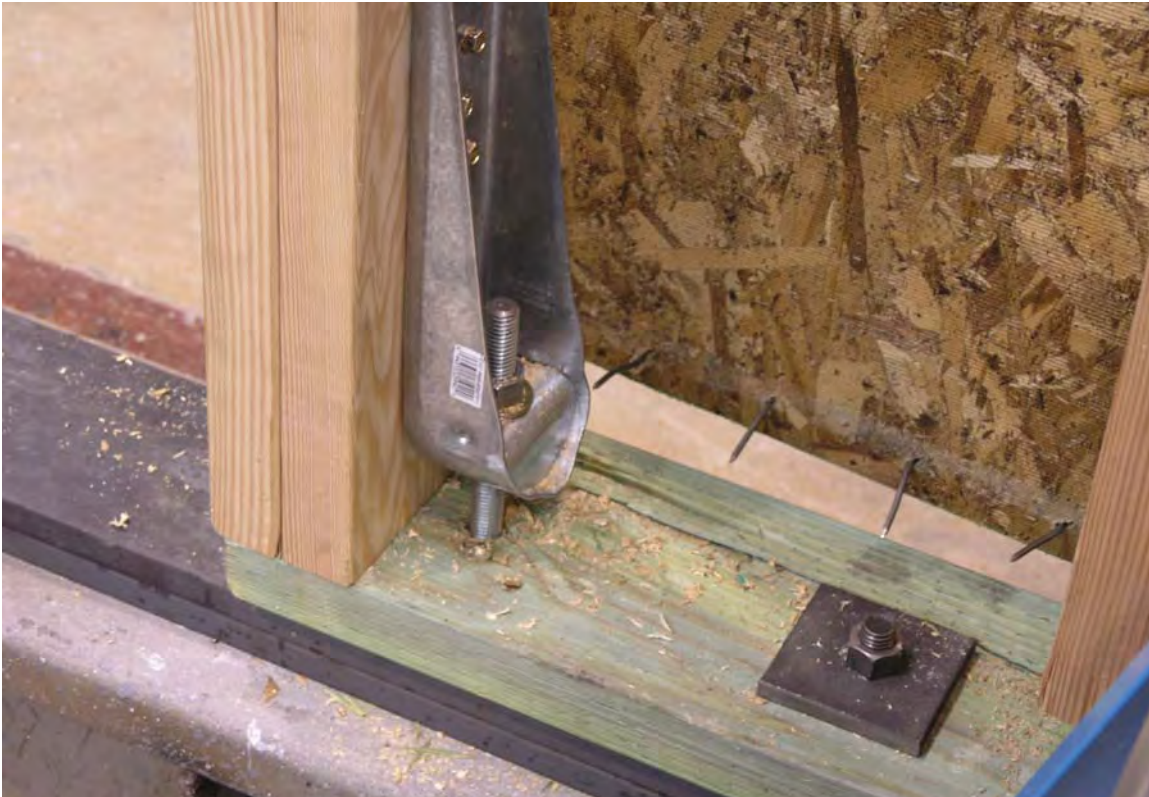
Figure 11. Separation of sheathing and splitting of bottom plate (Wall F1)
