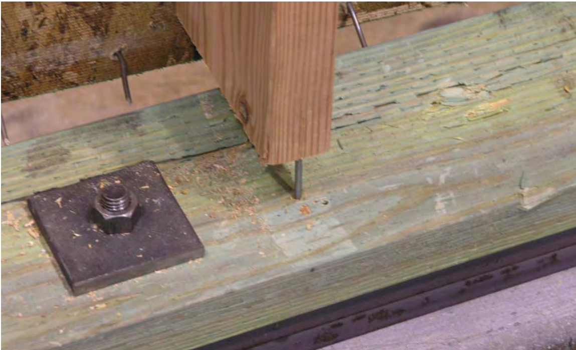
Figure 12. Splitting of bottom plate to the outside of square plate washer (Wall F1)
