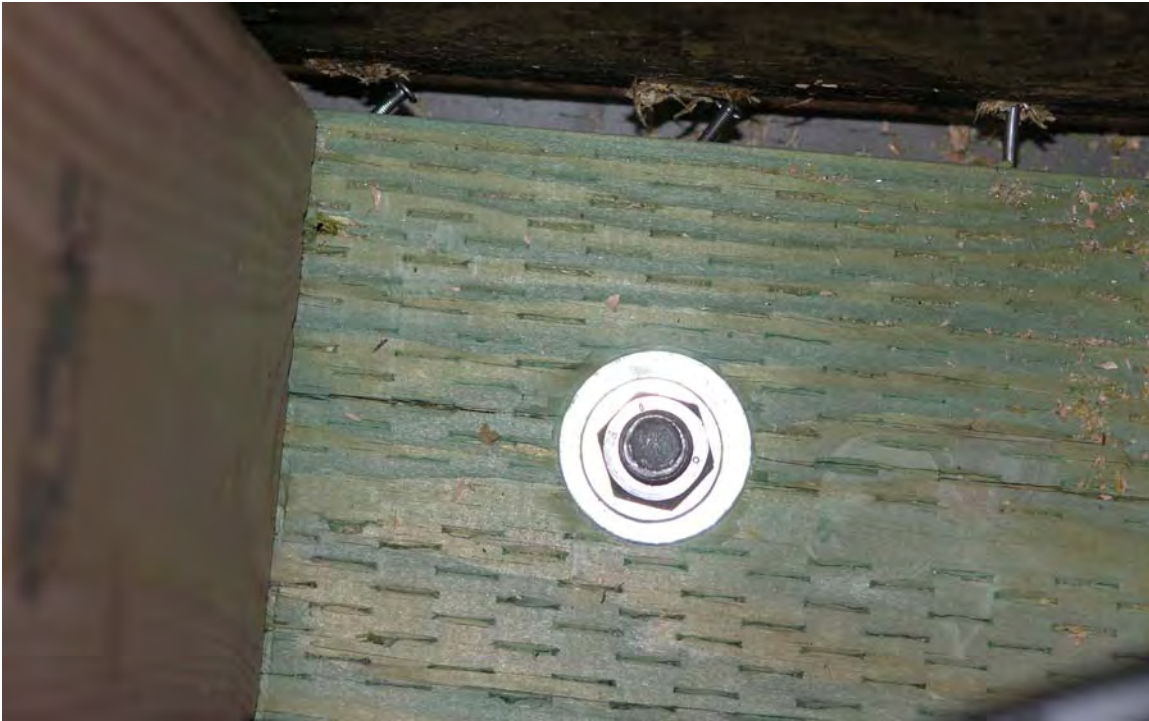
Figure 9. Splitting of bottom plate and separation of sheathing (Wall E2)
