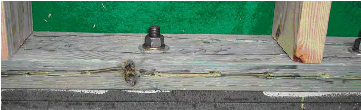
Figure 14. Splitting along narrow face on west side of wall (Wall G2)
