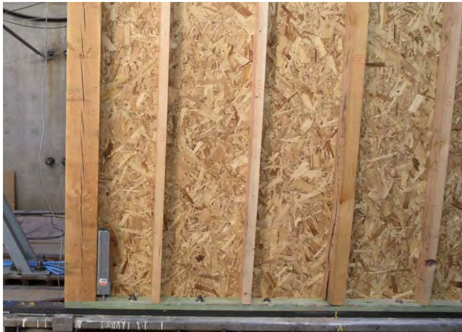
Figure 19. Wall H1 after testing.
