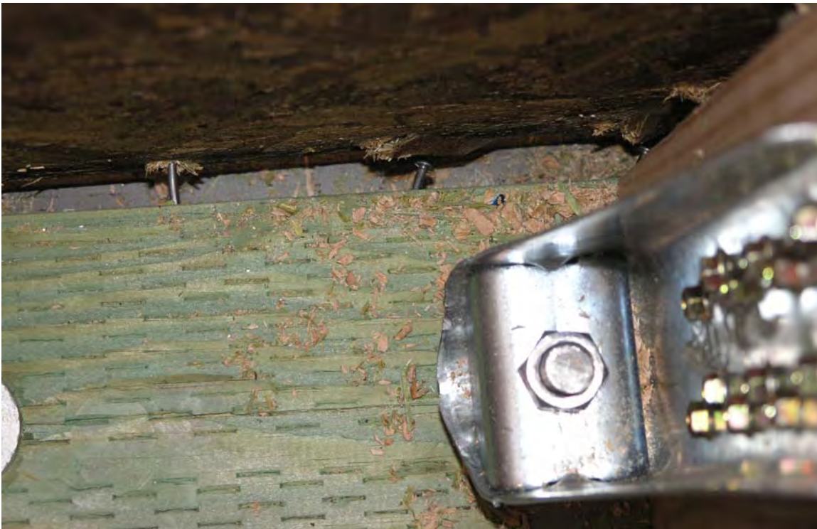
Figure 10. Splitting of bottom plate and separation of sheathing (Wall E2)
